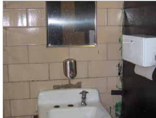
Besides sloppy paint on the tiles, the bathroom at MacArthur Park in Staten Island is in good shape. Maintenance issues such as broken sinks and needed repairs are the most common problem in park bathrooms.
