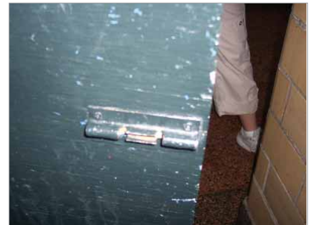
The lock on this stall door at Macombs Dam Park in the Bronx is broken, requiring maintenance.
